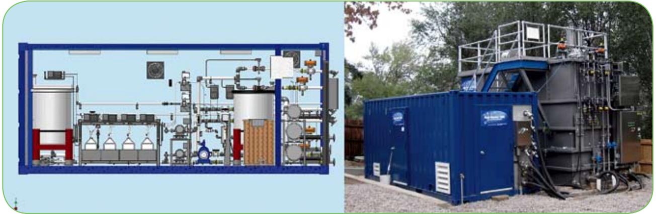
Figure 3. SBR-MBR Decentralized Installation at Colorado School of Mines
